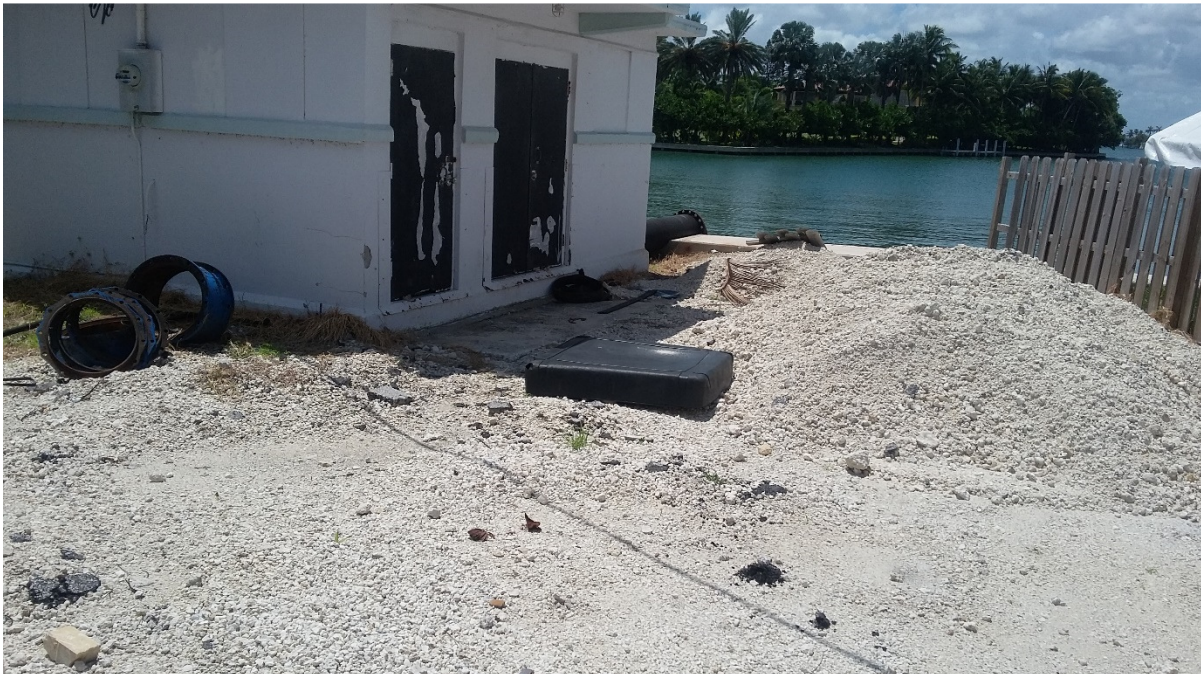
EXISTING PUMP STATION AT 92 ND STREET, CURRENTLY NOT IN SERVICE
