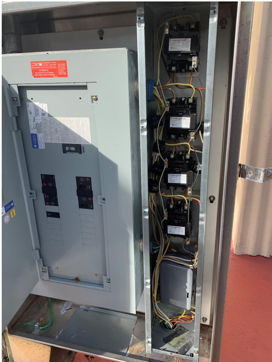
Panel inside enclosure
