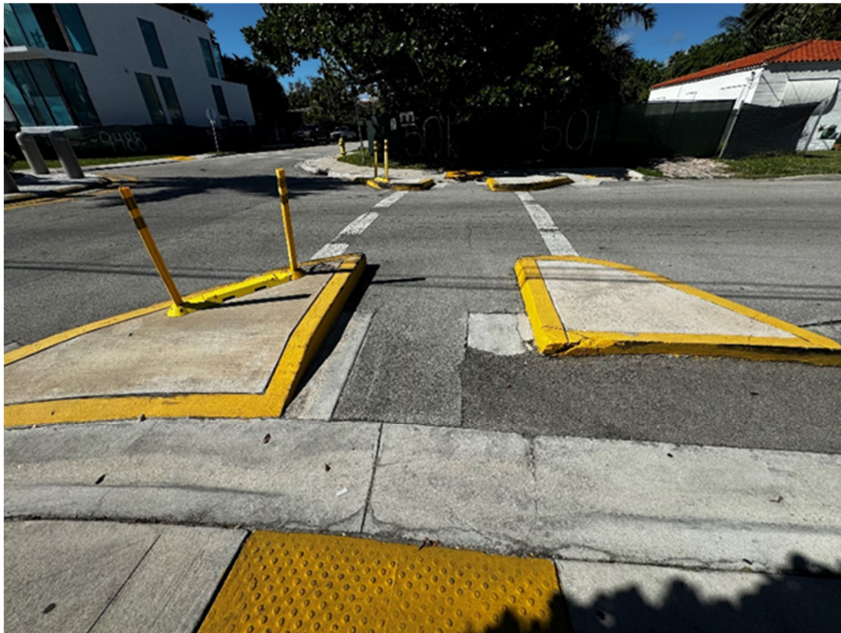
Figure 18 Existing Bulb out and crosswalk on Byron Avenue north of 95 th Street
