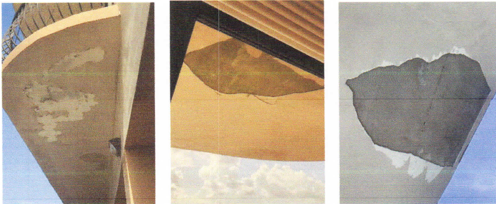
Figure D: Balcony Soffit paint spalling in units 208, 703, & 1301.
