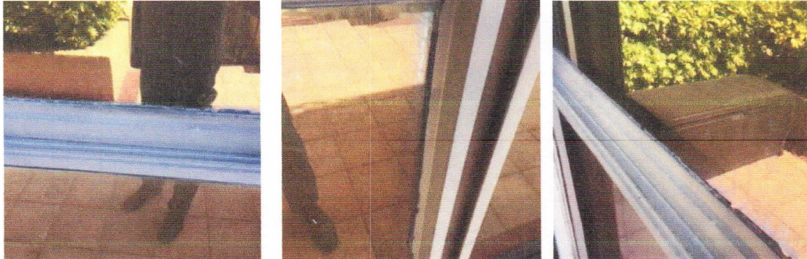
Figure F: Exterior sealant at window frame that has aged past its serviceable lifespan
