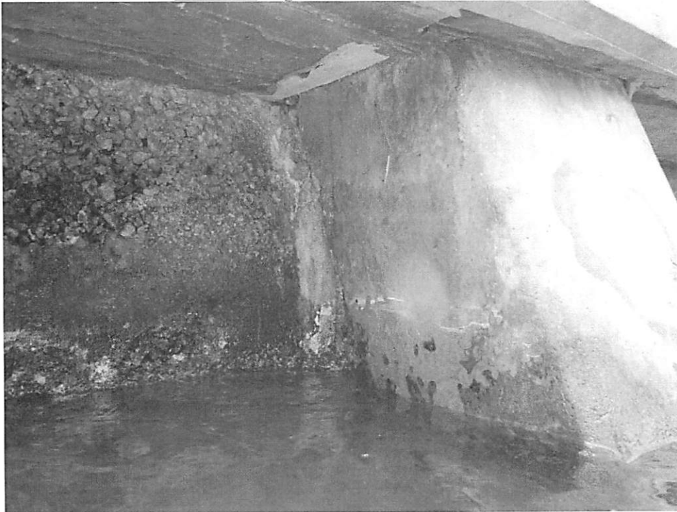
Photo 5.4: Degraded Concrete Sheet Piles
