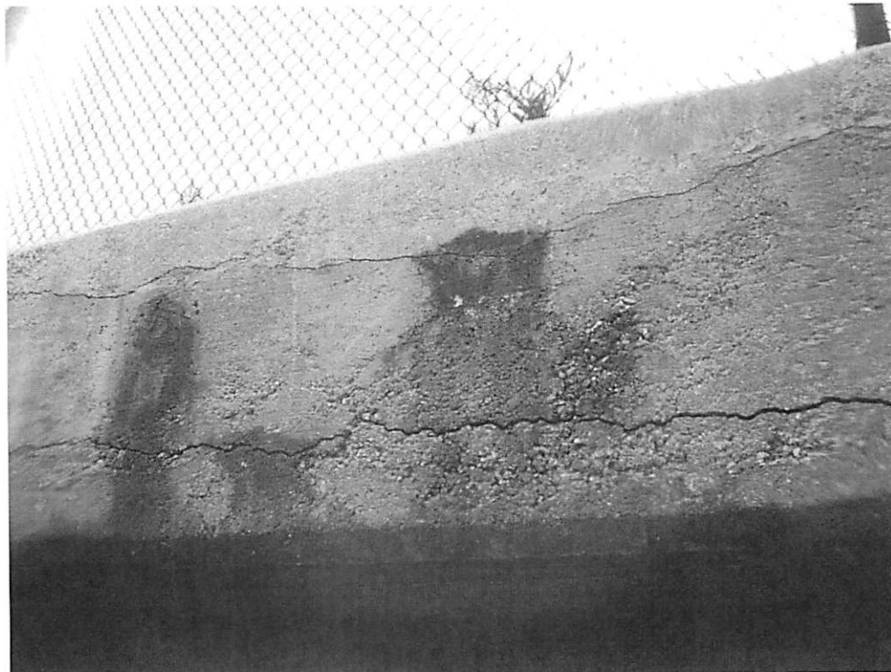
Photo 12.4: Longitudinal Spall Cracking in Cap, Rusted Reinforcement
