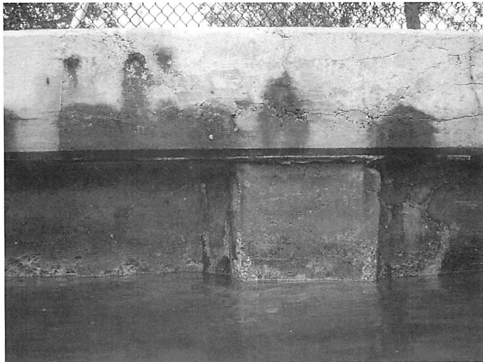
Photo 12.6: Longitudinal Spall Cracking in Cap, Rusted Reinforcement
