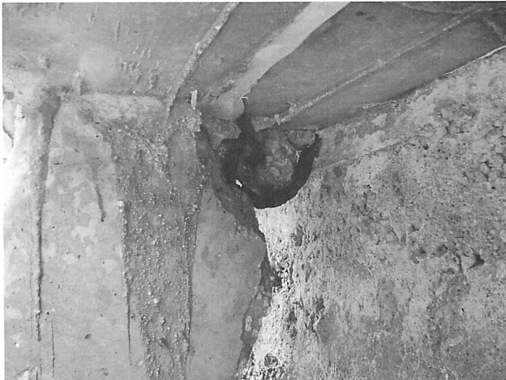
Photo 5.2: Exposed Steel Reinforcement in Batter Pile
