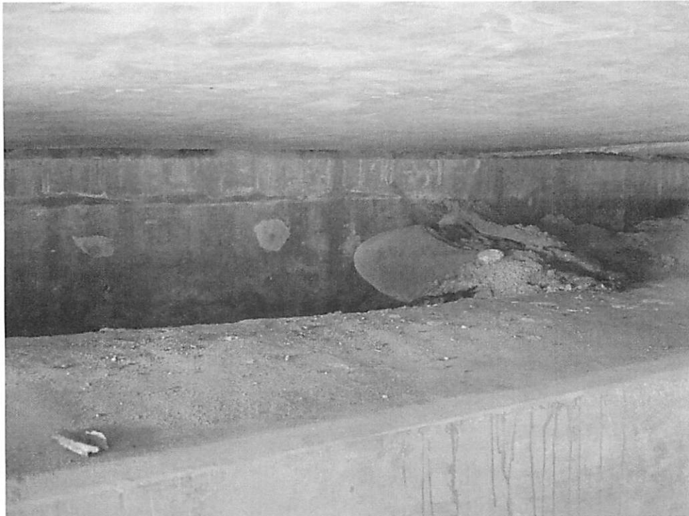
Photo 4.1: Sunken Area between Concrete Bulkhead and Bridge Abutment
