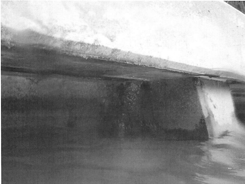
Photo 6.1: Exposed Steel Reinforcement
