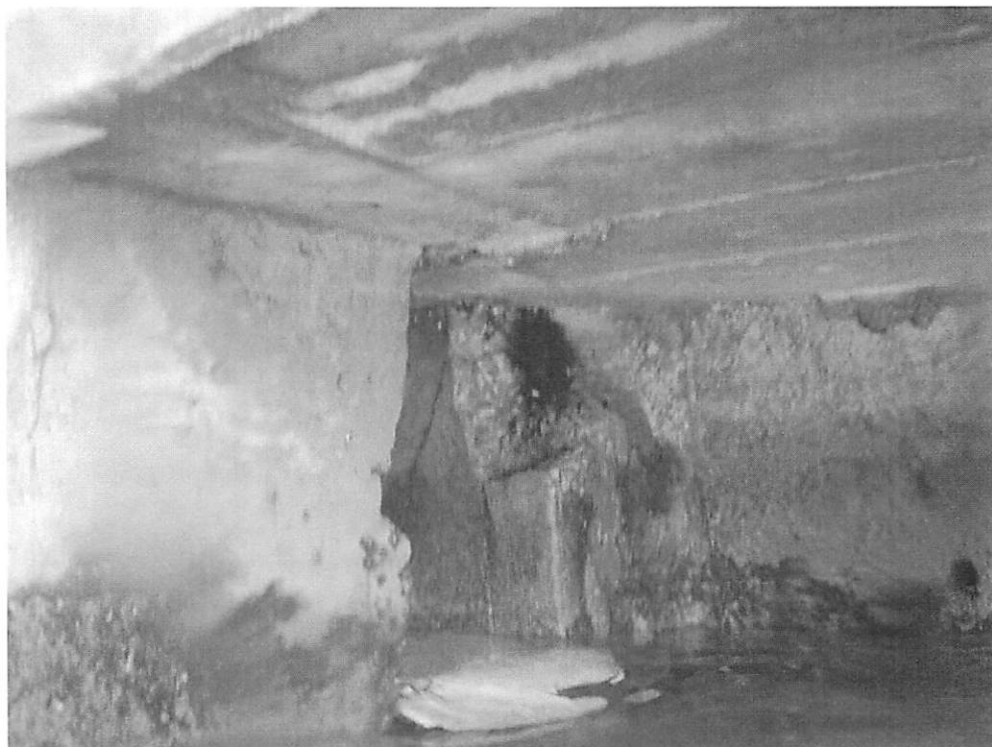
Photo 6.2: Exposed Steel Reinforcement
