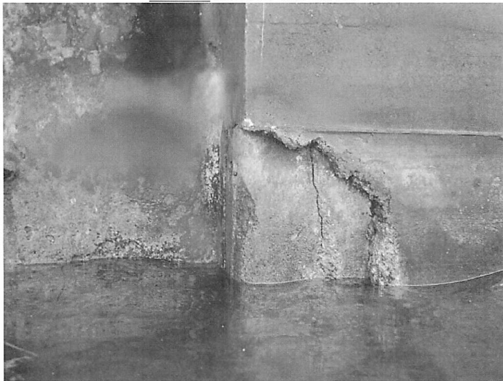
Photo 8.2: Cracks Observed in H-piles
