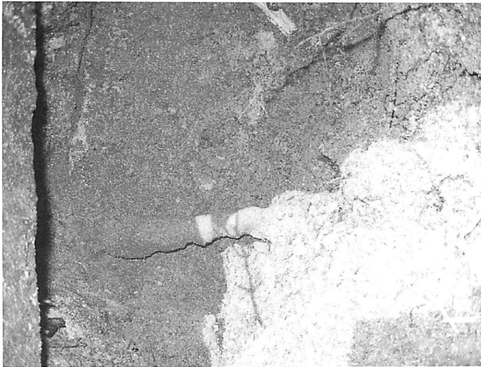
Photo 12.3: Excavated Tieback Rod in Good Condition
