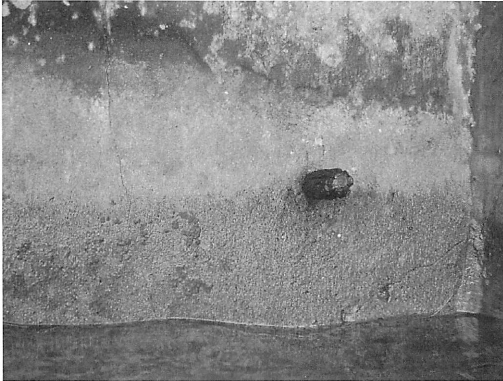
Photo 8.1: Rusted Tie-back Rod End
