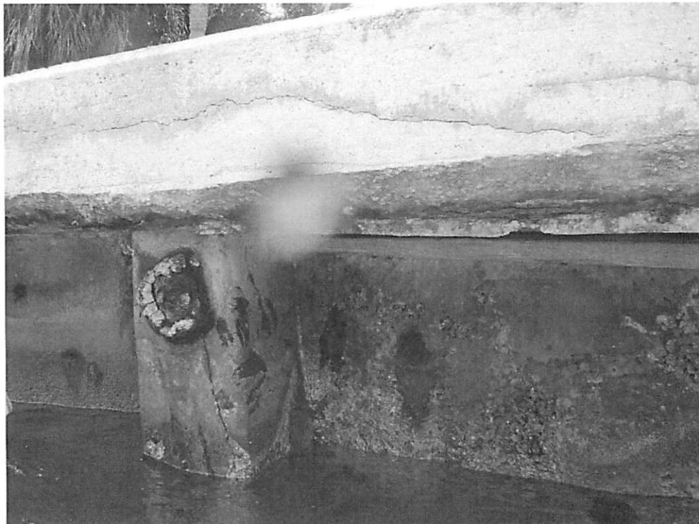
Photo 11.4: Cracking in King Pile & Cap, Degraded Sheet Piles
