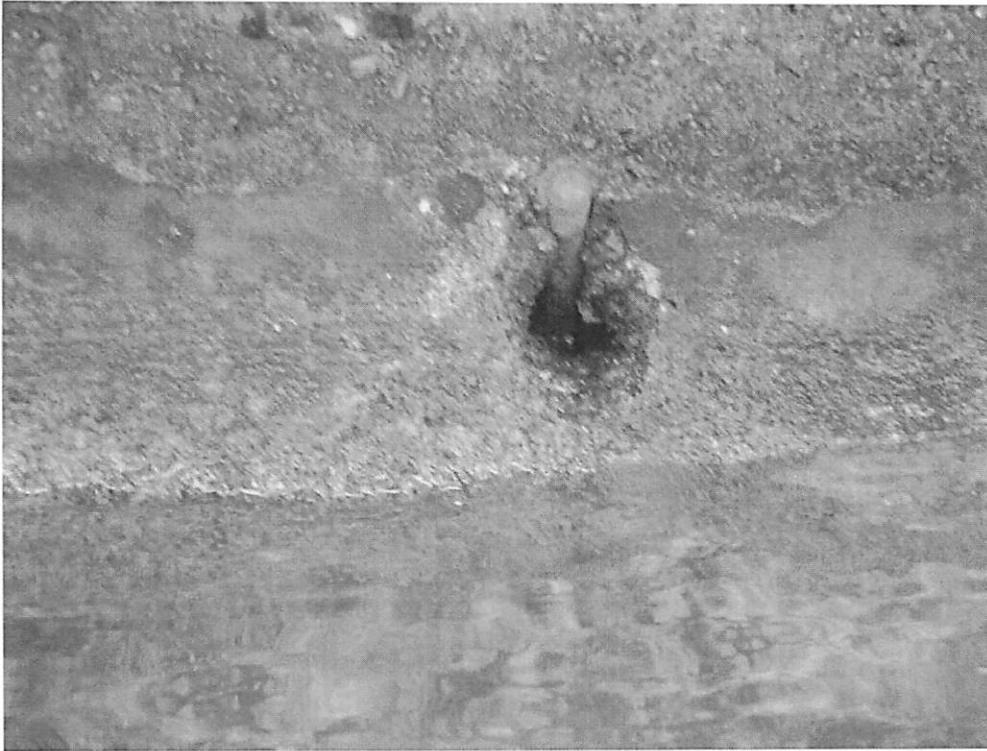
Photo 5.1: Tie Rod Pulled Through Sheet Pile
