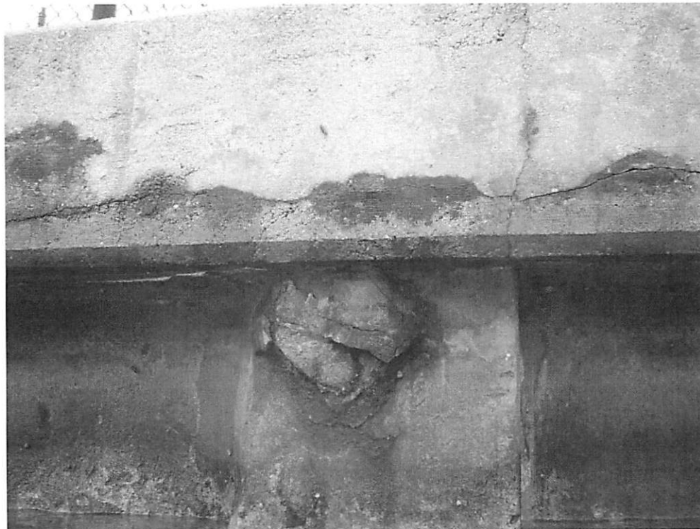
Photo 12.2: Longitudinal Spall Cracking in Cap, Rusted Reinforcement
