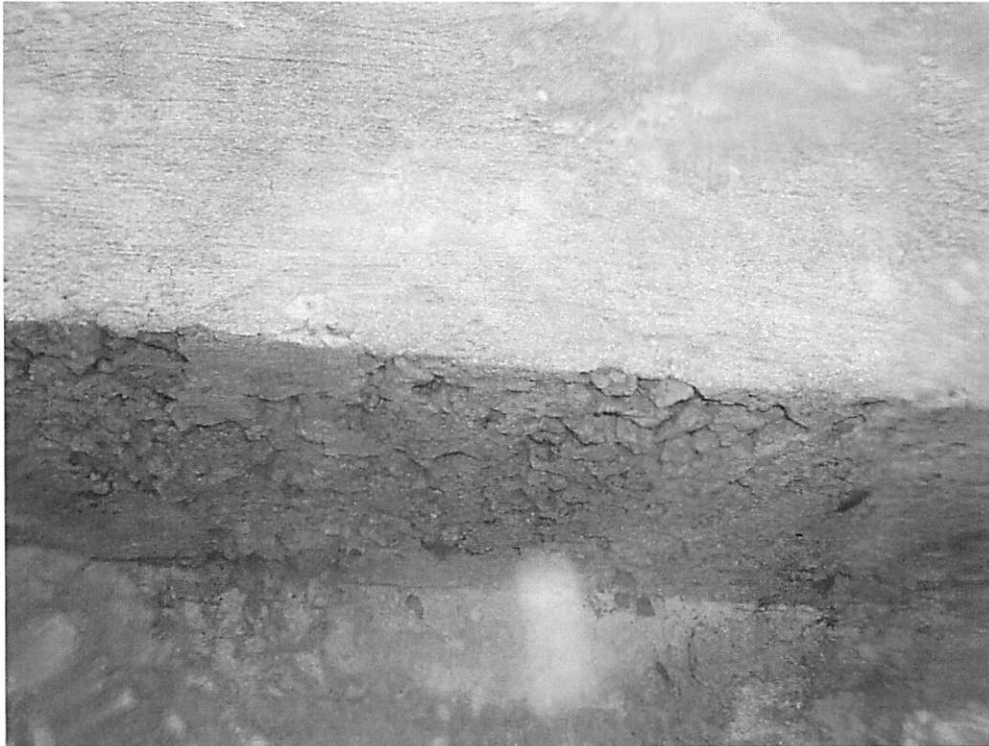
Photo 9.1: Honeycombing in Concrete Cap
