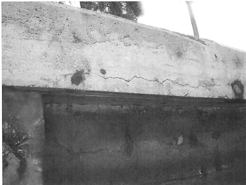
Photo 11.6: Spall Cracking in Cap, Rusted Reinforcement
