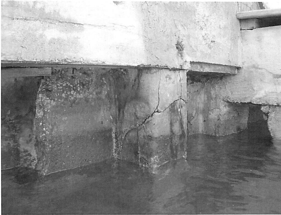
Photo 11.1: Cracking in King Pile
