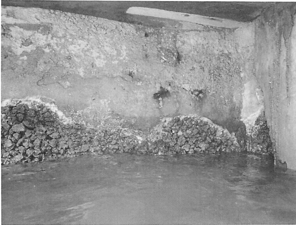
Photo 5.5: Degraded Concrete Sheet Piles
