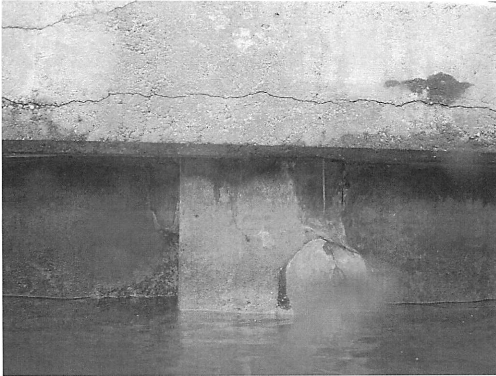
Photo 12.1: Longitudinal Spall Cracking in Cap, Rusted Reinforcement, Tieback Not Centered
