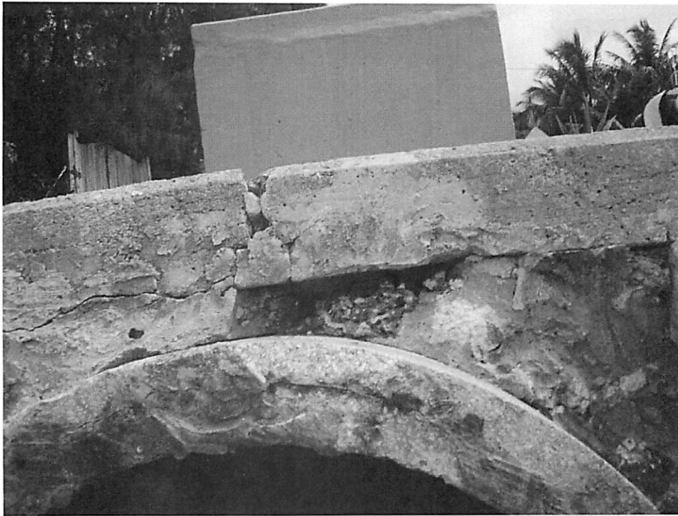
Photo 1.2: Crack above Concrete Outfall
