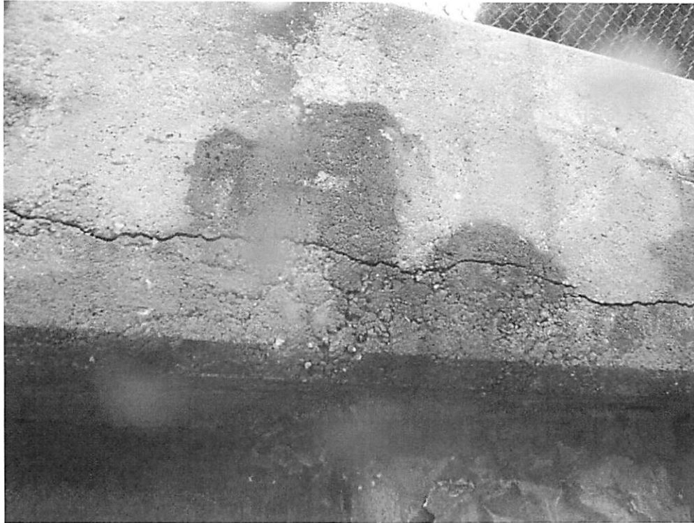
Photo 12.5: Longitudinal Spall Cracking in Cap, Rusted Reinforcement
