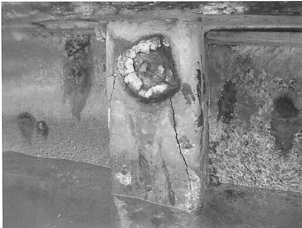
Photo 11.2: Cracking in King Pile, Spalling Cap
