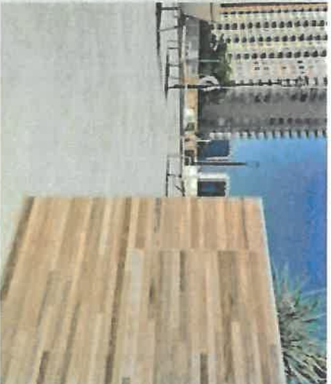
The amenities area received a new porcelain deck and wood-look mosaic planters.
