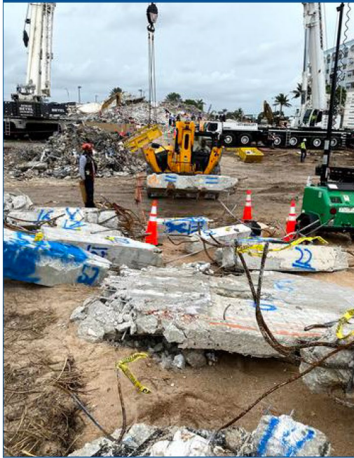
Building elements such as columns, beams, and floor slabs identified for evidence review (July 2021)
