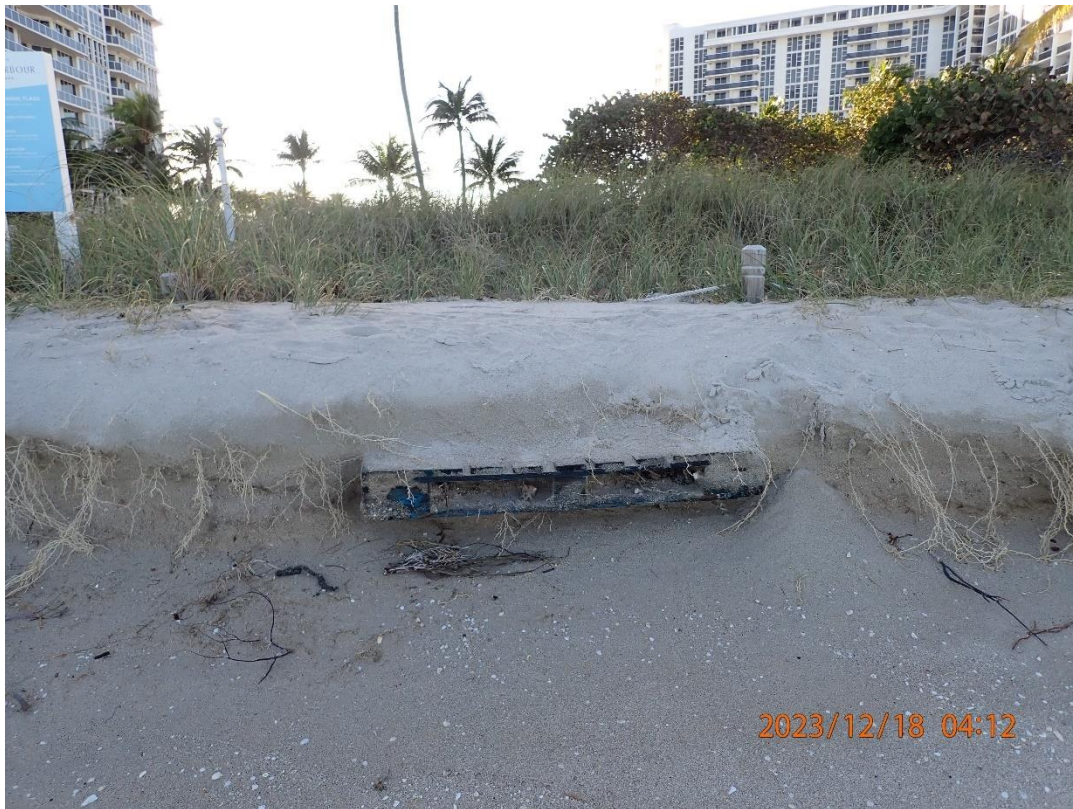
PHOTO 19. EXPOSED WOODEN PALLET AT DUNE SCARP NORTH OF ACCESS 18
