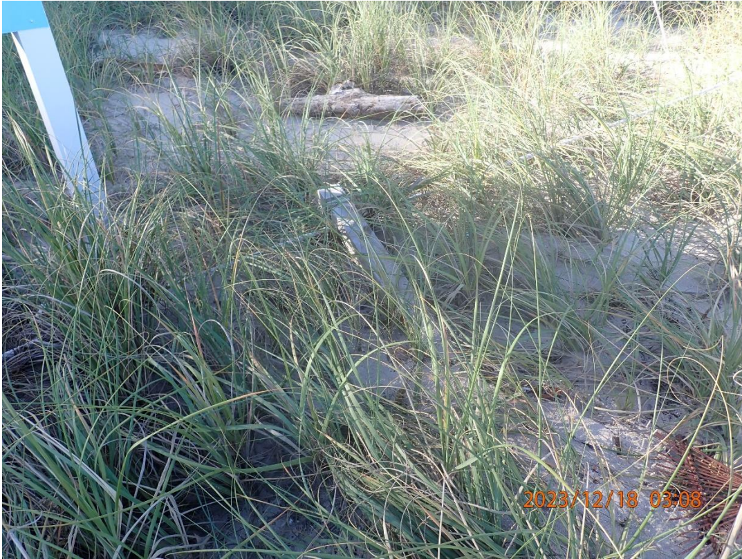
PHOTO 8. DOWNED FENCE POST NORTH OF ACCESS 11
