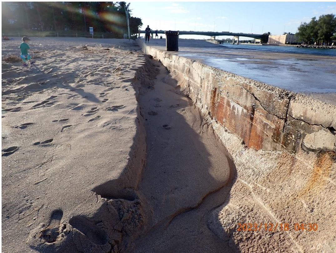
PHOTO 21. SEDIMENT EROSION SOUTH OF JETTY
