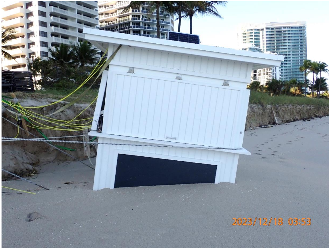
PHOTO 16. MAJOR SETTLEMENT OF ACCESS 15 BEACH KIOSK
