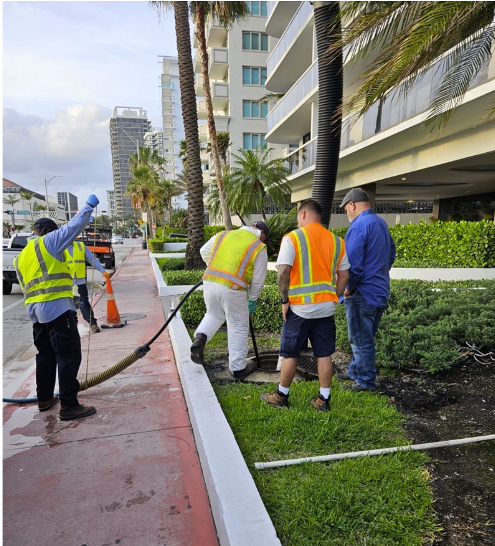
Backup at 9455 Collins Avenue
