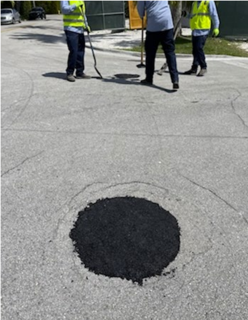
Patched potholes throughout Town
