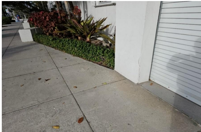
CRACKS OBSERVED AT DOOR JAMB
