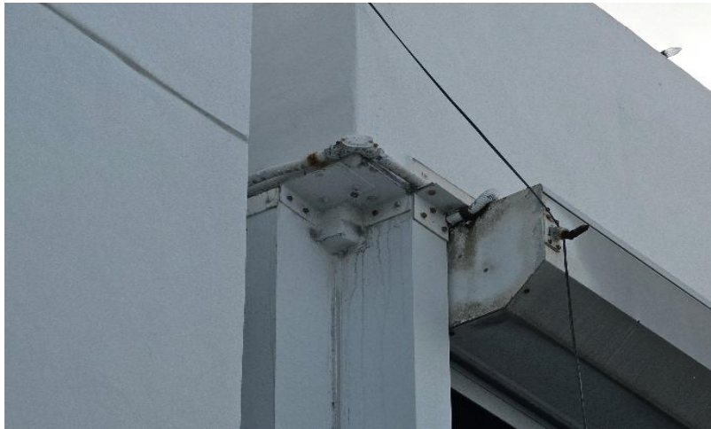
RUST OBSERVED ON EAST ENTRANCE STOREFRONT FRAMING
