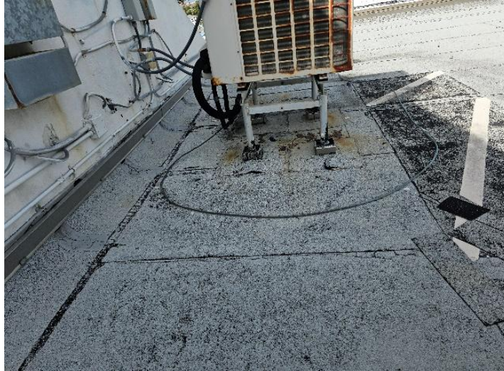
RUST OBSERVED AT RTU BASE CONNECTION
